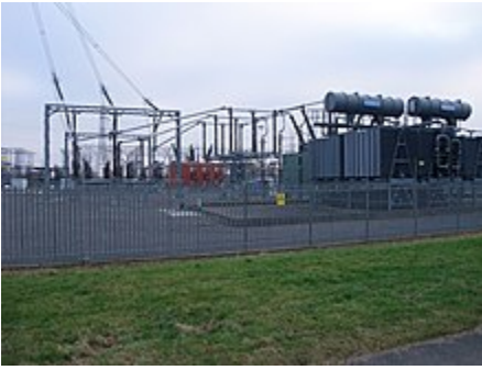
A Grid Transformer Station
