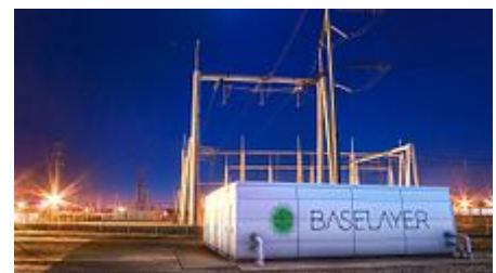
A modular data center connected to the power grid at a utility substation
