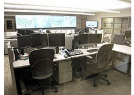
Overview of a typical NOC. Status monitors (front), backbone overview (back), and news broadcast on TV-set (right). Note safe under desk, typically for backups, passwords, or hardware cryptographic devices. - Picture of the Global Network Operations Center [GlobalNOC] at Indiana University
