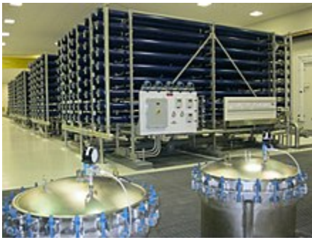
Reverse osmosis production train, North Cape Coral Reverse Osmosis Plant
