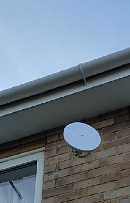
A CableFree CPE Radio installed for Rural Internet in The Cotswolds, UK
