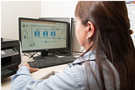
Example of SCADA used in office environment to remotely monitor a process
