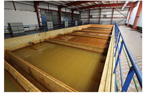
Tanks with sand filters to remove precipitated iron (not working at the time)
