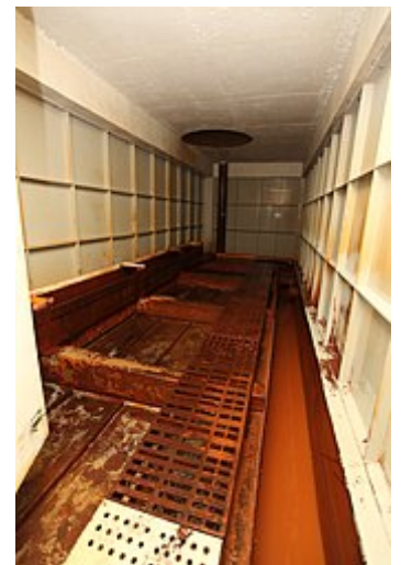
Empty aeration tank for iron precipitation
